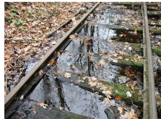
Drainage through the rails at Rt. 28 cut
